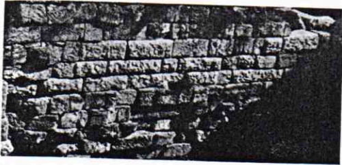
Undercutting of a wall due to dissolution of its building stones, Eleusis site
