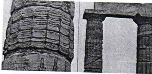
Weathered and cracked columns and slabs, Temple of Poseidon, Sounion site
