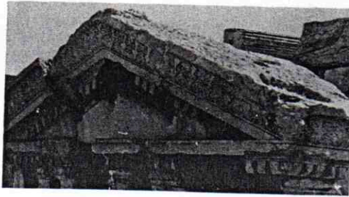
Chemical and mechanical weathering of an ornamental architectural member, Eleusis
